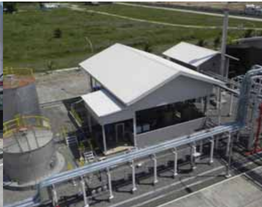
Boiler and demin plant (Jun '13)
