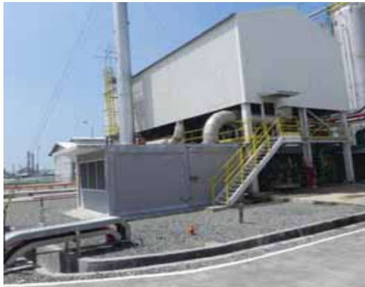
Compressor house (Jun '13)
