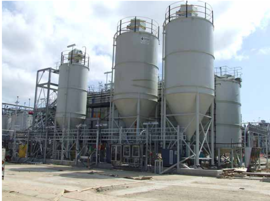
Mining chemicals installations
