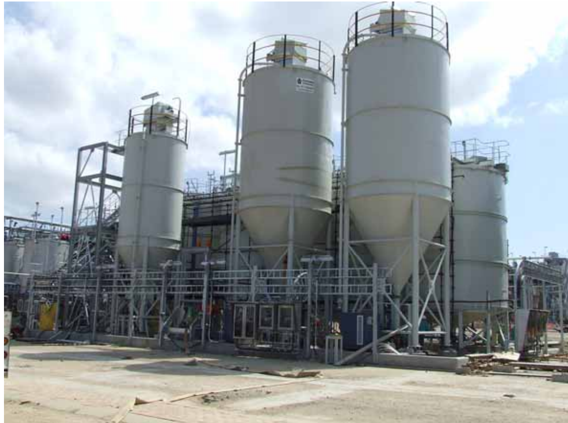
Mining chemicals installations
